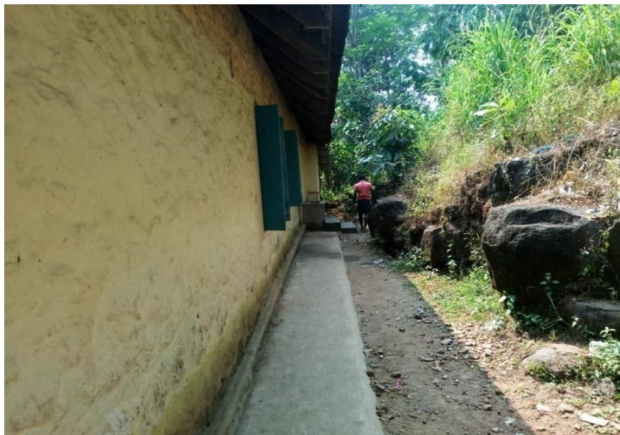
Boundary wall needed to restrict the water from the mountain
